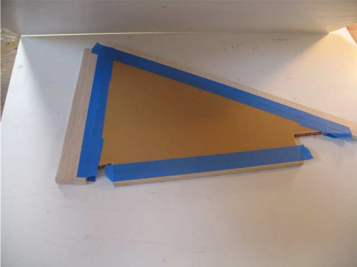
Using the tape as a hinge I opened up the joint and applied Aeropoxy. The edging is then closed and tape applied. Both sides of the joint are sealed with tape.
